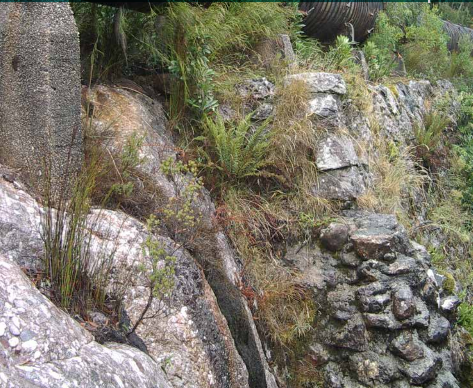
Lake Margaret Power Scheme, Queenstown
