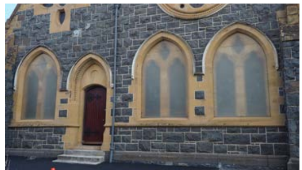
Church of the Apostles (THR 4206). Windows prior to works commencing with Perspex coverings with no stained glass visible from the window. Credit - Hans Wander.
