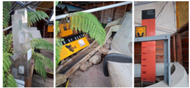
Hydro-electricity infrastructure installation © NRE 2024
