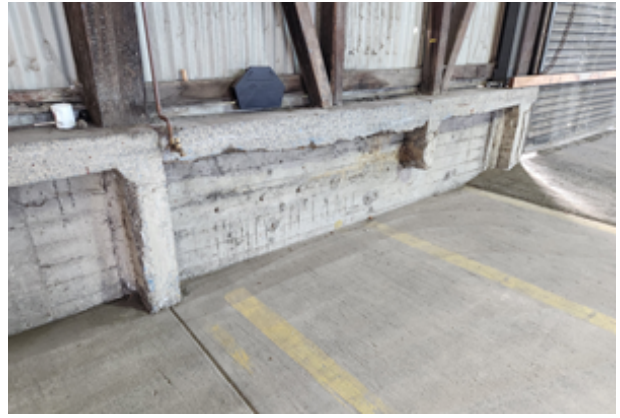
Broken concrete slab-edges and stubs of former sub-floor walls within the Shed's northern end.
