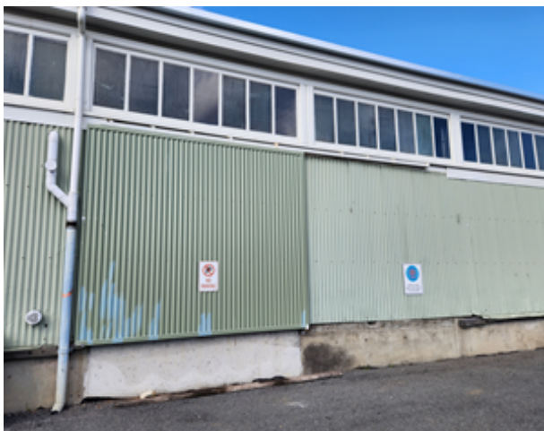
The sole remaining externally-mounted head-track at a former sliding goods door opening. © NRE Tas Aug 2023
