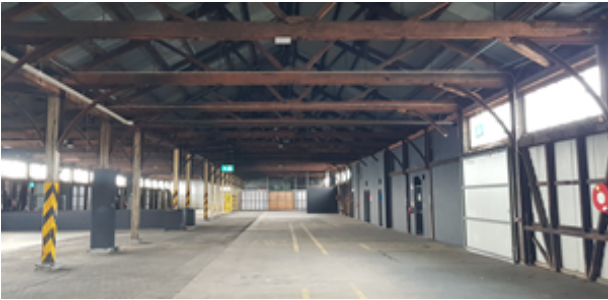
Paving changes from concrete slabs to segmental pavers at the edges of former loading platforms.
