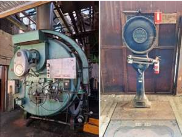
Northern section: disused boiler; scale © NRE 2025
