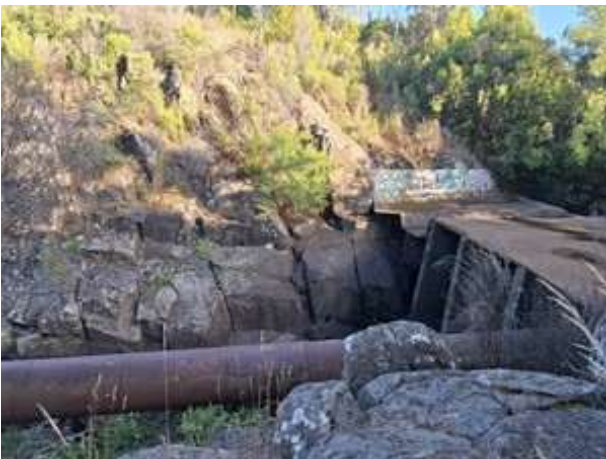
Water supply pipe: Distillery Creek weir © NRE 2026
